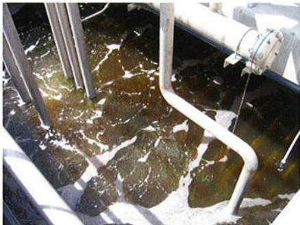
Final disposal site leachate treatment facility 最终处理场 渗透水处理设施
