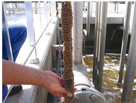
Leachate treatment facility Condition of attached sludge in the aeration tank 渗透水处理设施 硝化槽污泥附着状态
